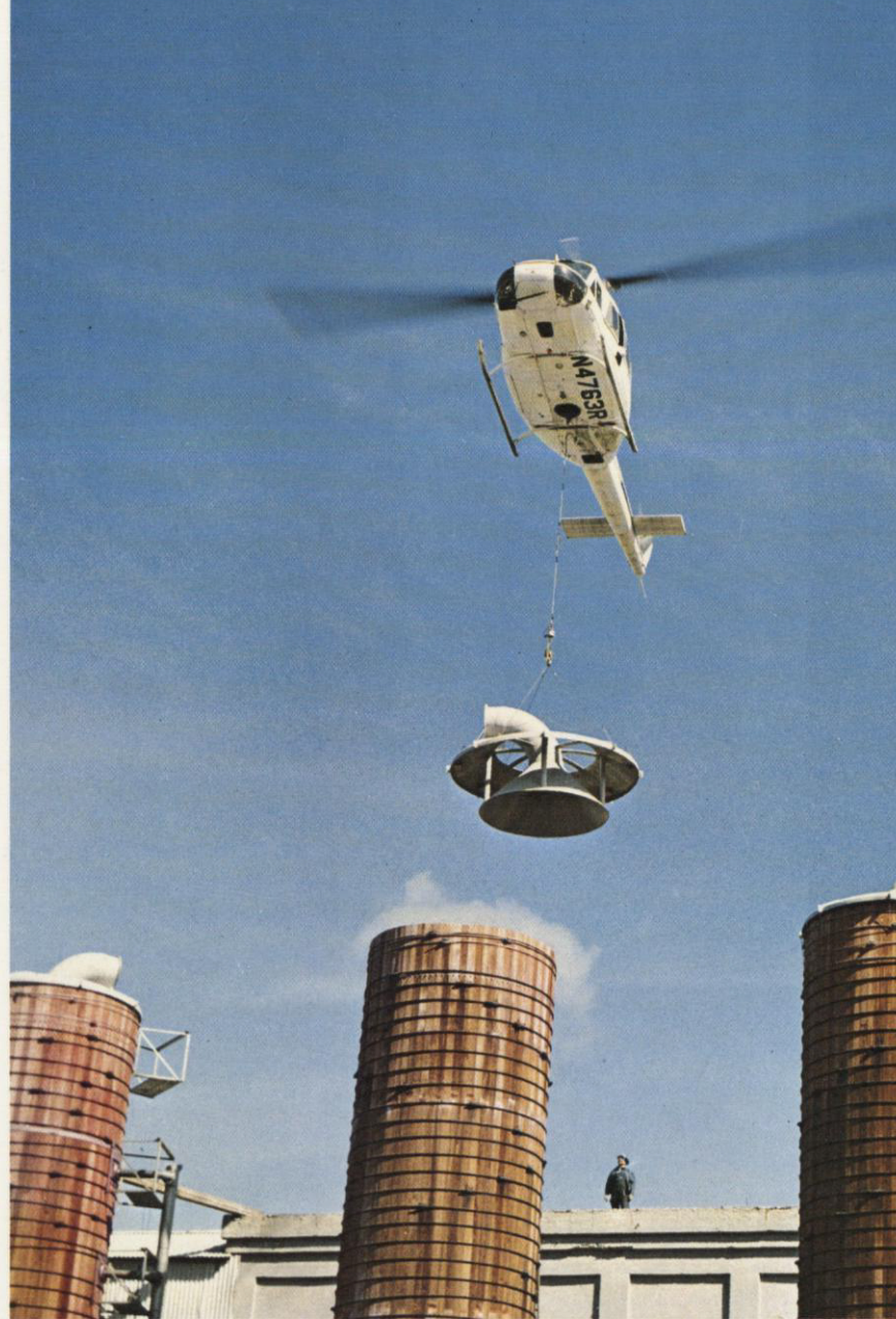
Above: Helicopter lowers antipollution "digester cap" into place on gas recovery tower at an ITT Rayonier mill in Hoquiam, Washington.
