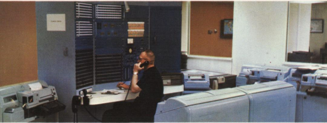
Control console of automated terminal station, for continual monitoring of U.S. State Department transmission circuits, is part of store-and-forward message switching system for which ITT Defense Communications is the prime contractor.
