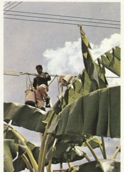
Below: Lineman of ITT's Puerto Rico Telephone Company at work helping to carry out the company's five-year expansion program calling for 125,000 new telephones throughout the fast-growing Caribbean commonwealth.
