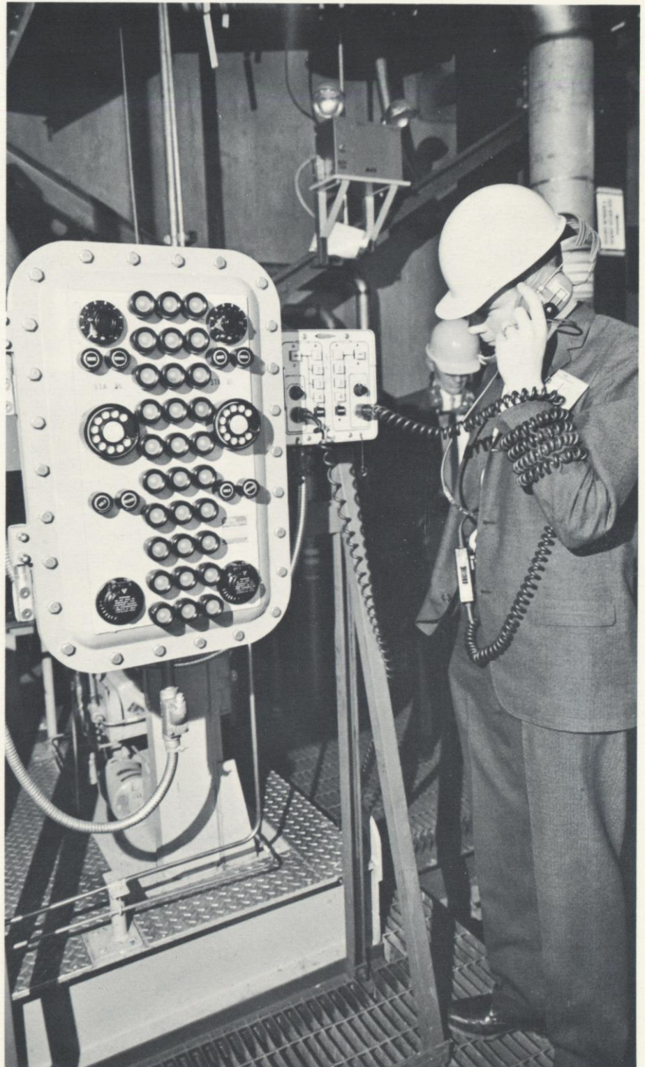
An ITT engineer conducts one of many performance tests of an explosion-proof communications panel for the launch maintenance conference network in an Atlas "F" series missile silo in Oklahoma. ITT is the prime contractor to the U. S. Air Force for ground communications in the Atlas program.
