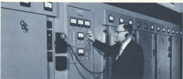
LTV's 50-kilowatt commercial broadcast transmitter fills FCC requirements for unattended operation of radio equipment.
