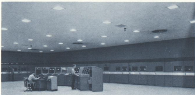
Control consoles for world's largest radio station simplify operations, insure reliability of continuous communications.
