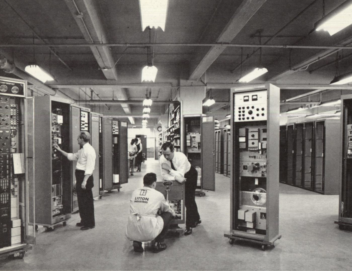
POINT-TO-POINT COMMUNICATIONS UNITS ARE ASSEMBLED AND TESTED BY ENGINEERS IN THE NEW YORK CITY FACILITIES OF THE WESTREX CORPORATION DIVISION
