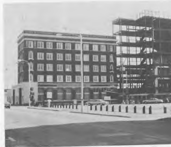
Old Swedish-American Bank Building at left; at the right is the new structure going up behind the old. The old building will be razed.
