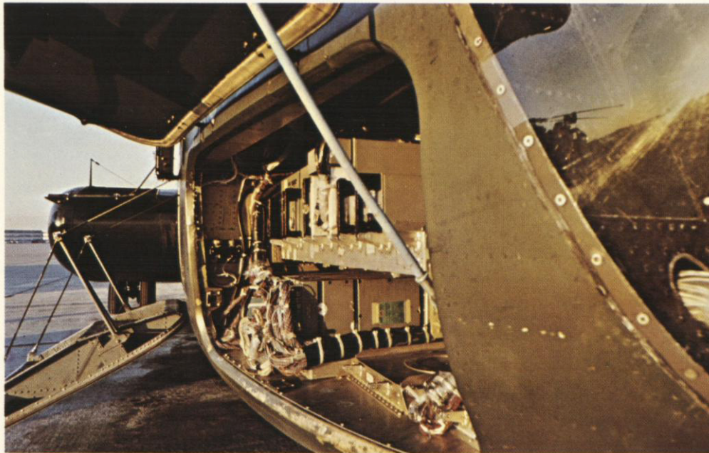
Equipment components of the Integrated Helicopter Avionics System (IHAS) are visible in one of the electronics compartments in a CH-53 helicopter.
