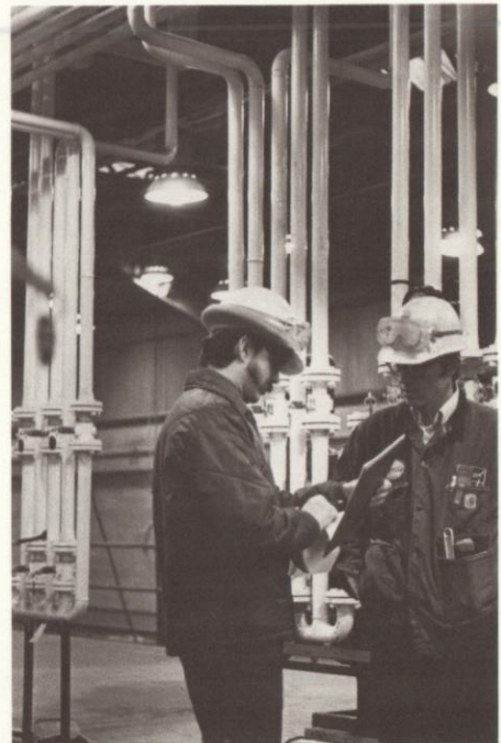
Intricate piping systems carry raw materials from storage to production reactors.
